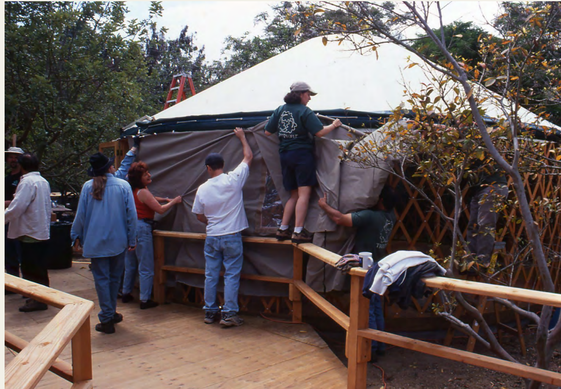
TreePeople staff gather for a “yurt raising” to create office space in an old orchard. (2003)
