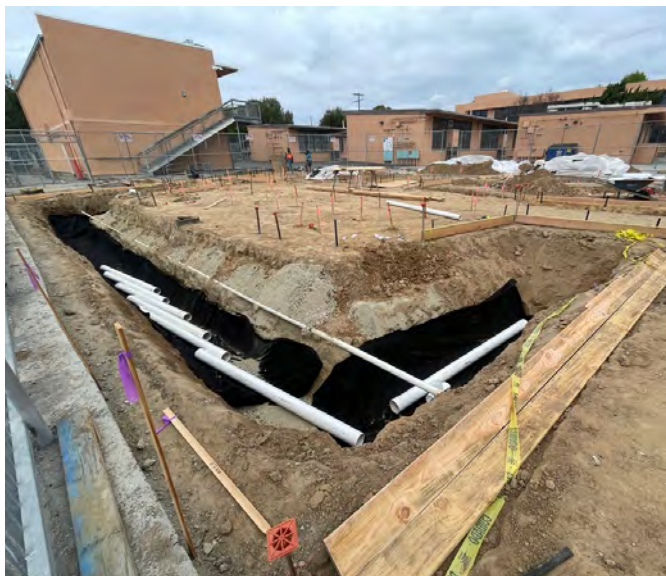
Wilmington Middle School stormwater infrastructure system
